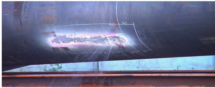
1 – Leak on a pipeline
